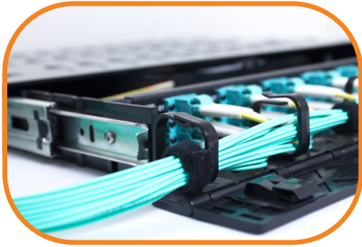
Front Patch Cable Management
